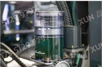
润滑系统 Lubrication oil pump system
